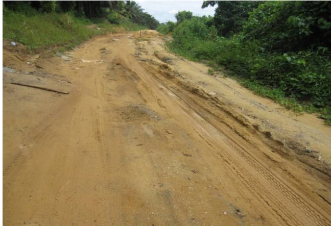
Infrastructure routière difficilement praticable
