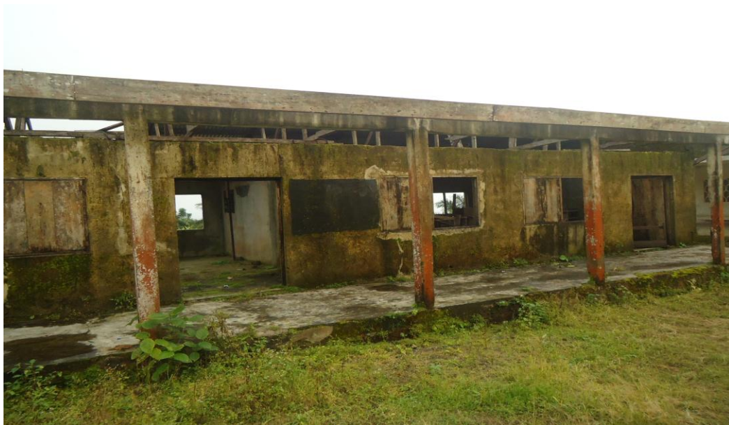
A. Dilapidating G.S, roof blown off by storm.
